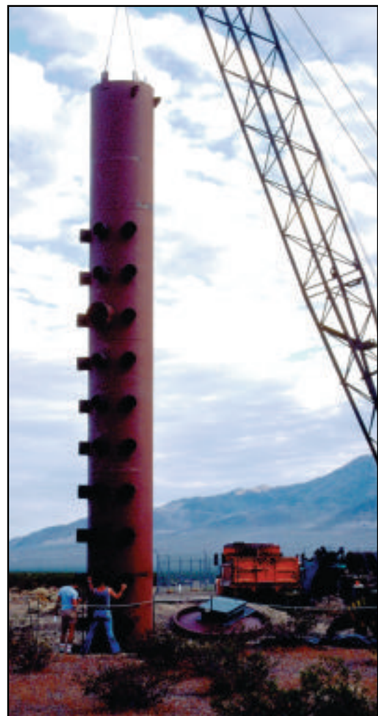
Figure 4. Installation of vertical shaft used for soil-moisture monitoring in upper 45 feet of unsaturated zone beneath undisturbed, vegetated area. Photograph by David S. Morgan, U.S. Geological Survey, August 1983.
